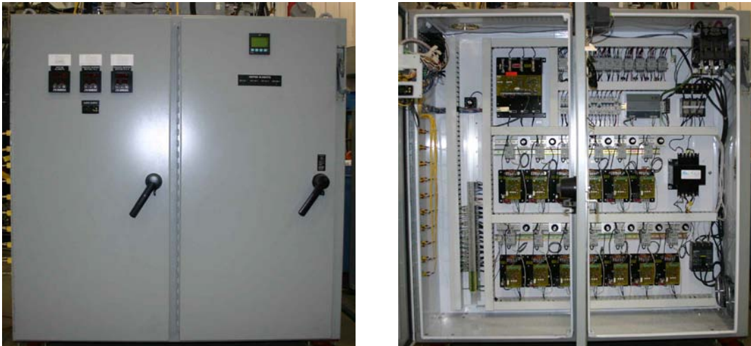
Figure 15. Heaters Power Control Cabinet
