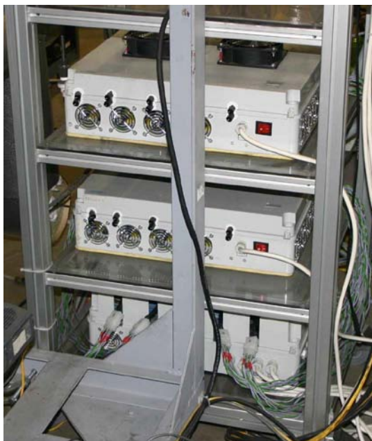
Figure 22. Capacitors (Lower) and Converter (Two Upper) Modules.
