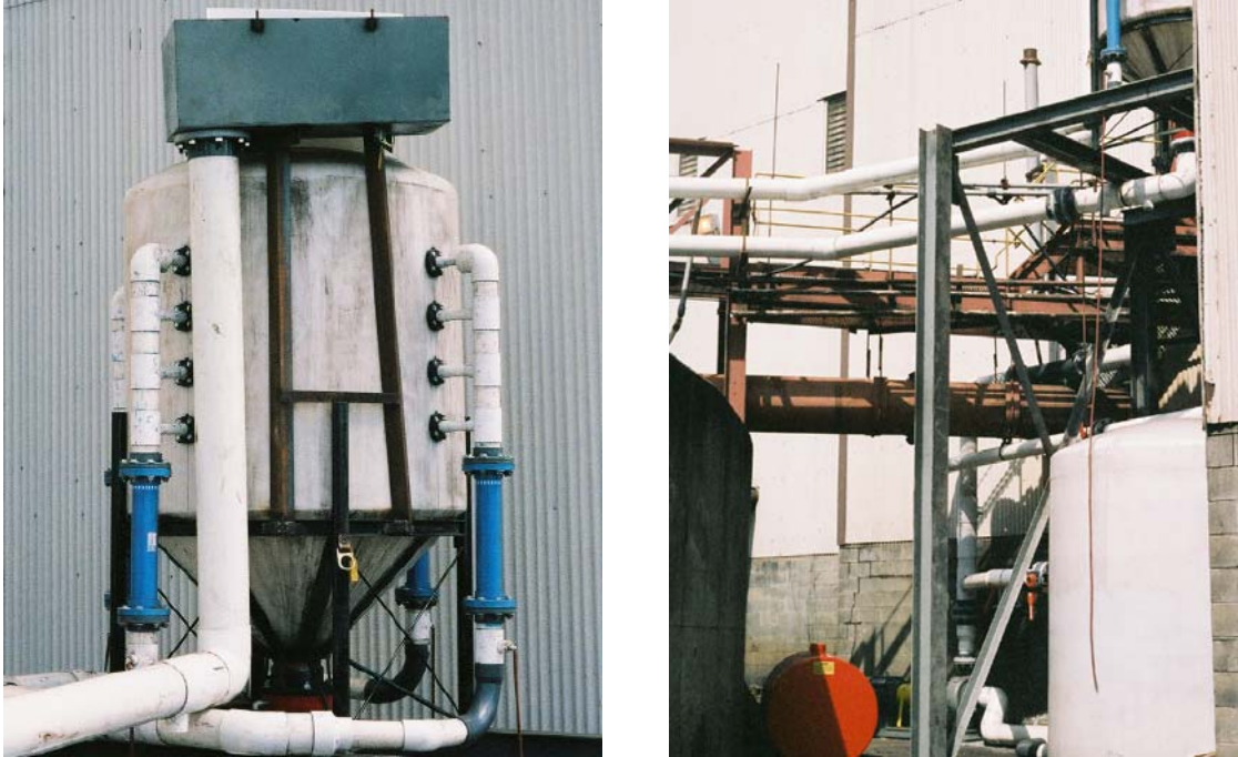
Figure 4. MRC Installation at Freeman Energy Demonstration Site
