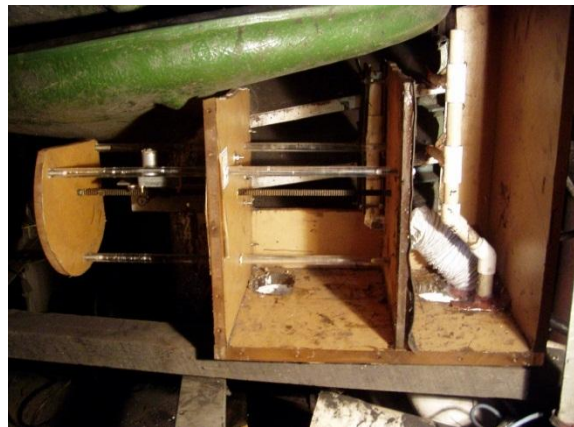
Figure 26: New robust splitter box installed in Creek Paum plant.
