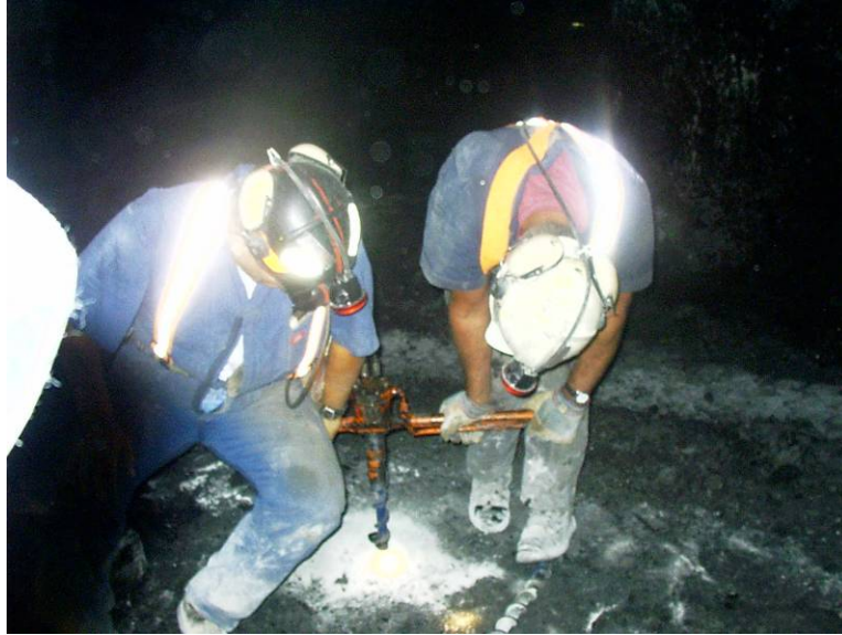
Figure 5. Installing convergence points by drilling into the floor using a Schroeder drill.
