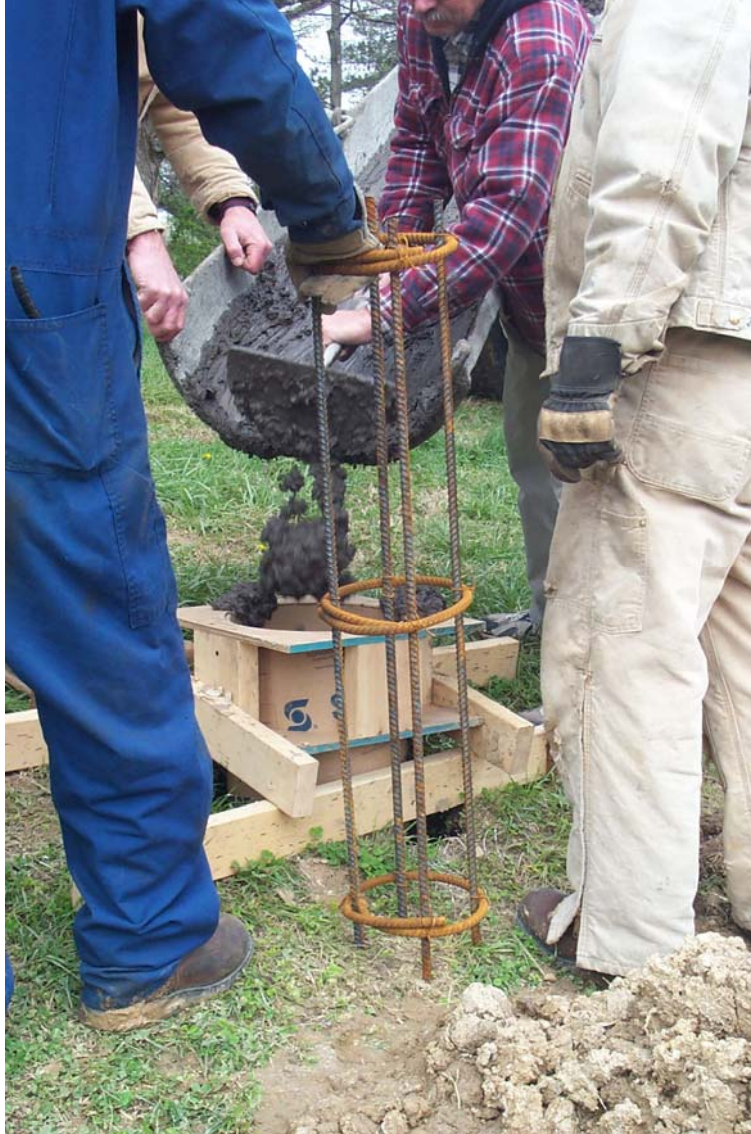
Figure 6. CCBs based foundation pier being poured with the steel rebar ready for insertion.
