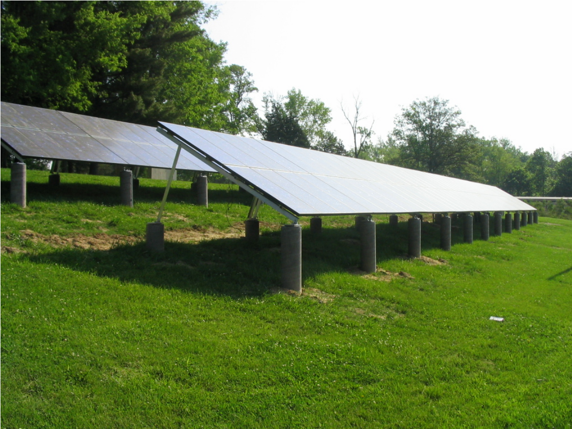
Figure 10. Photo-voltaic array deployment on CCBs based concrete foundation piers.
