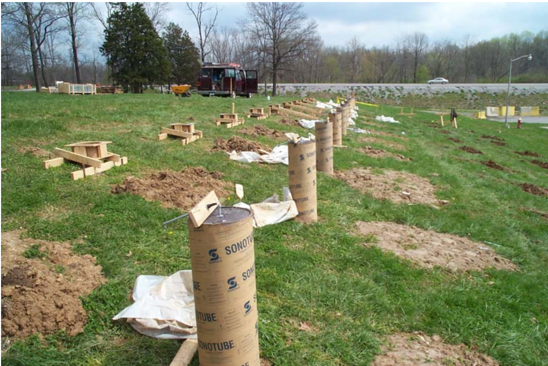
Figure 8. A row of twelve CCBs based foundation piers a few days after implementation. Forms for the second row of piers are ready and visible in the background.
