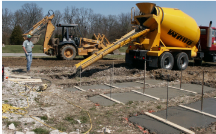
Figure 9. Construction of trenches for bond strength testing in progress RESULTS AND DISCUSSION
